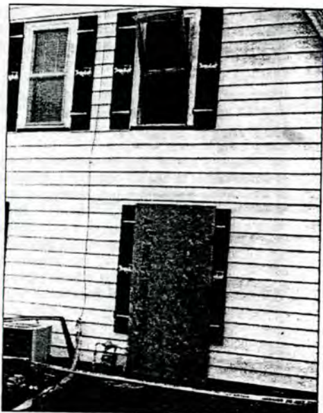
The Emma Lefeber home, 203 3rd Ave., Portsmouth, sustained extensive damage Monday. (Photo by Chad Goetsche)
